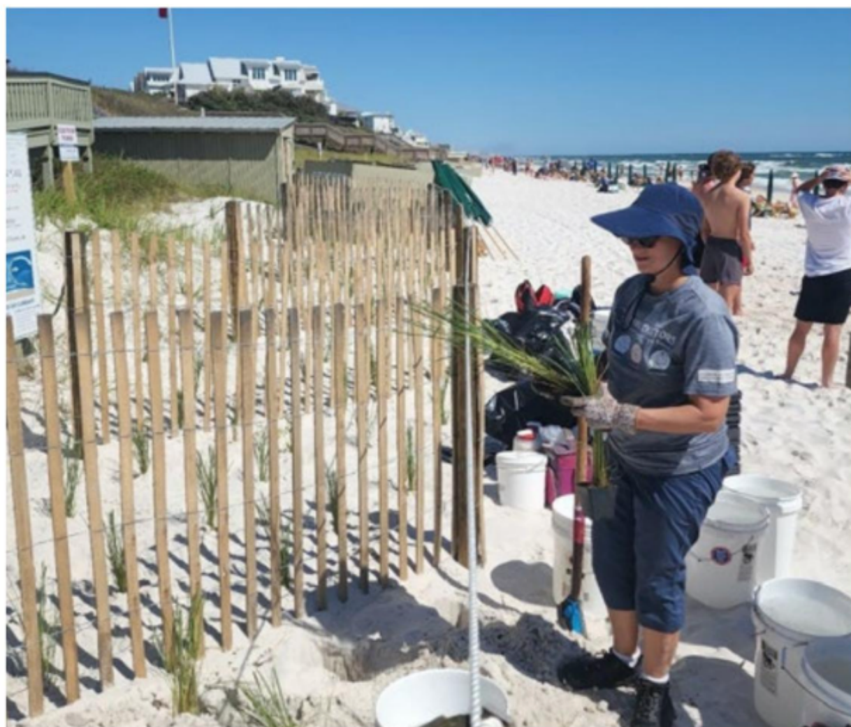
Frederique Beronet, MBA & MS Biology, installs sea oats to initiate a new protective berm.
